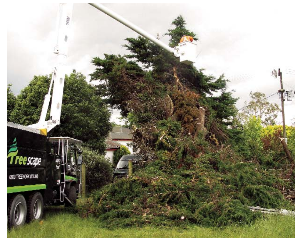
Nick Sprott makes the first cut on the contract by taking on a Cypress tree on Nichols Rd Road.
